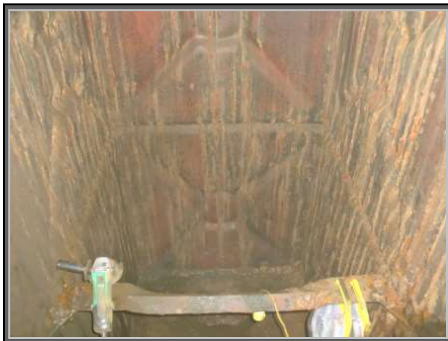
Internal corrosion of CWST 1 once drained
